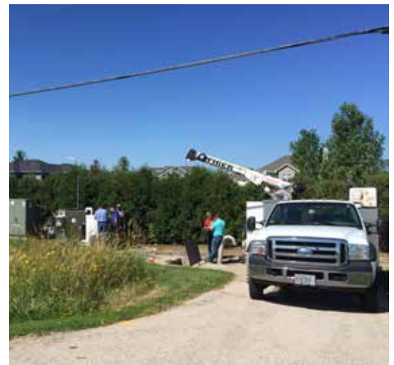
Fond du Lac lift station being upgraded with innovative Concertor™ pumping system.
