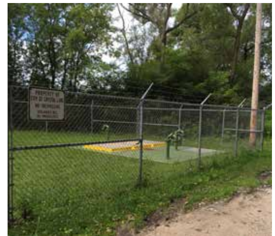
Crystal Lake pump station
